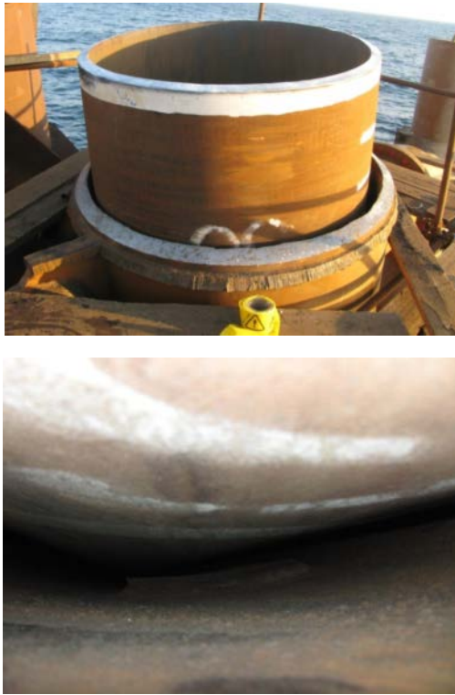
Fig. 2: a) Pile head of un-grouted piling system b) Wishbone element installed in un-grouted piling system
