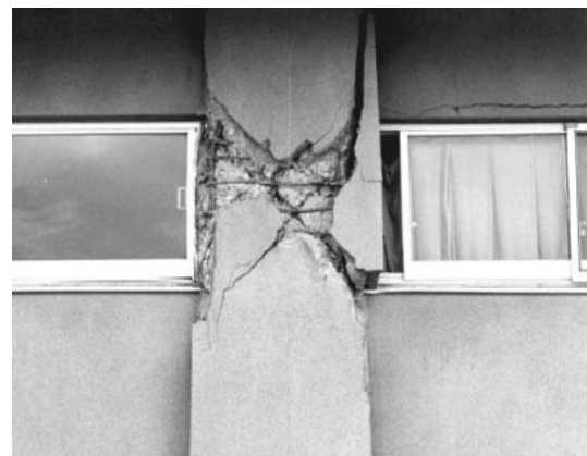
Fig. 16. Short column due to the partial infill wall, the 1987 Miyagi-Ken Oki (Japan) earthquake (Guevara and Garcia, 2005)
