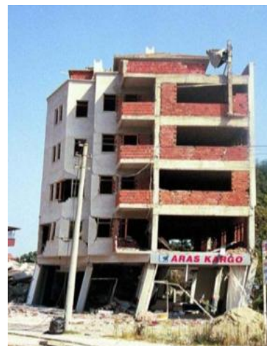
Fig. 13. Soft storey due to the elimination of masonry infill wall in ground floor, the 1999 kocaeli (Turkey) earthquake (Yatağan, 2011)
