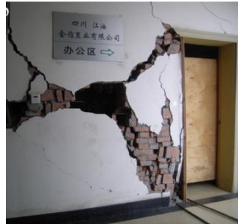
Fig. 4. Diagonal cracking and in-plane failure of wall, 2009 Wenchuan earthquake, China (Zhao et al. , 2009)
