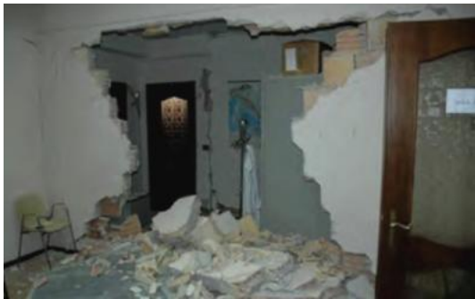
Fig. 7. Out-of-plane failure, of wall, the 2009 L'Aquila earthquake (Ceci et al. , 2010)
