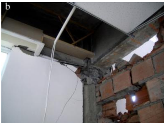
Fig. 19. Failure of wall corner and shear failure of column; the 2008 Wenchuan earthquake (Zhao et al., 2009)
