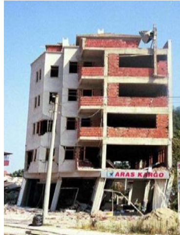
Figure 2. Soft storey in the 1999 kocaeli (Turkey) earthquake due to elimination of masonry infill wall in ground floor (Yata an, 2011)
